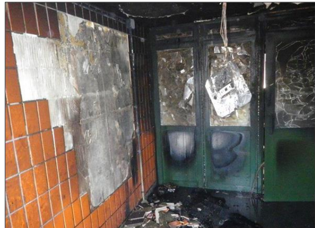
Image right: View from other side of doors. Note extensive damage to ceiling, walls, doors and wall panels. Light fitting and electrical wiring indicated by red arrow also damaged by fire.
