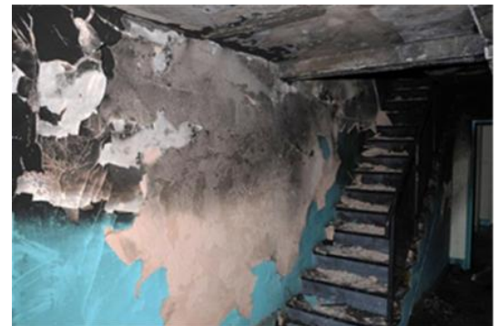
Stairwell opposite the scooter. Note: spalled plaster from the stairwell has fallen onto the stairs
