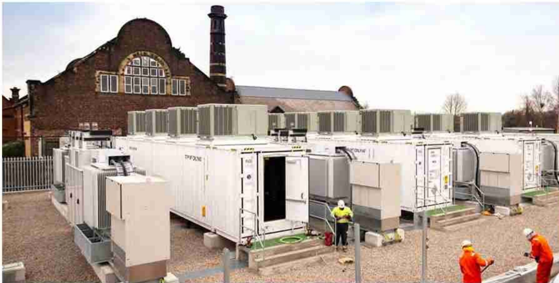
Figure 5 LiBESS installation on Merseyside that exploded in September 2020
