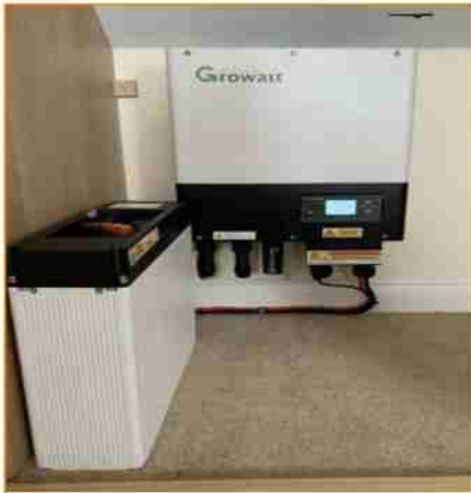
Figure 1 Small scale domestic BESS
