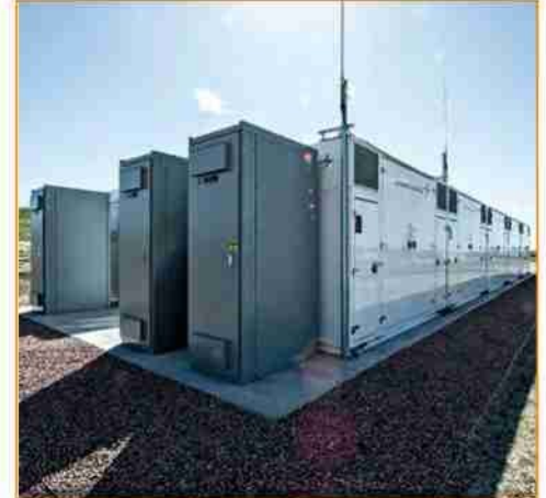
Figure 3 Industrial scale BESS
